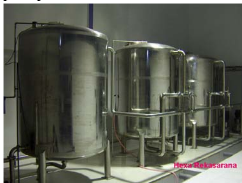
Gambar 3.8. Water Treatment Plant.
